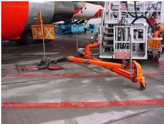
An example of a correct installation of a Hydrant coupler.
