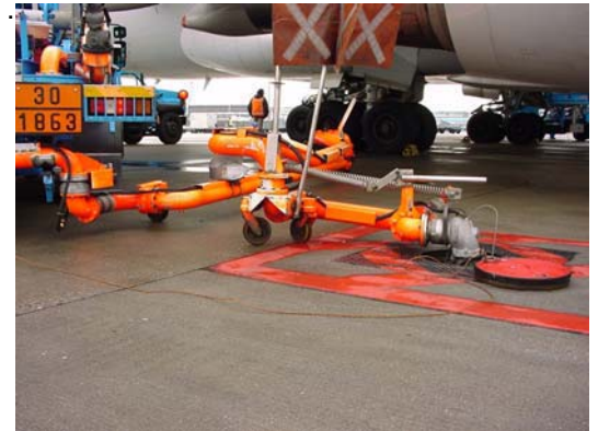
One example of a "Rigid Piping Assembly" showing an incorrect installation.
